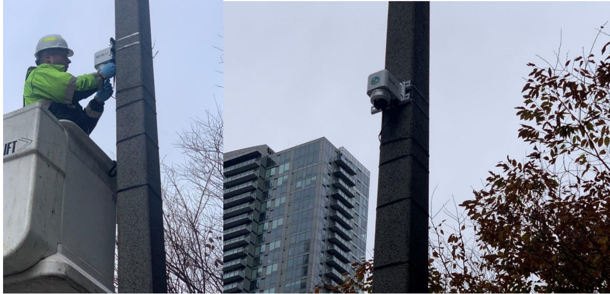
Figure 5-7 MUST Sensor Installed in Bellevue Test Bed
