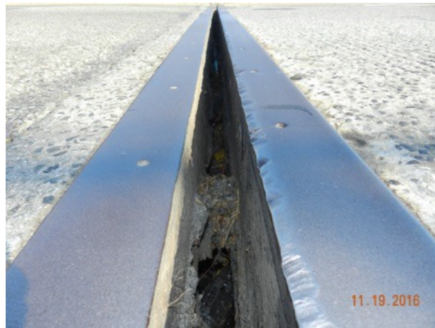
Figure 11: Missing Compression Joint Seal
